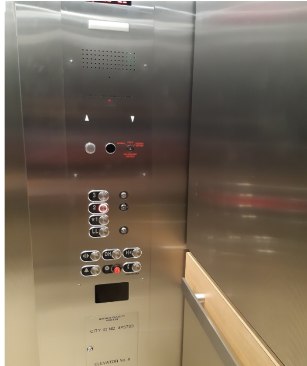
Elevator # 8 in the F-Corridor, one of many back in service
